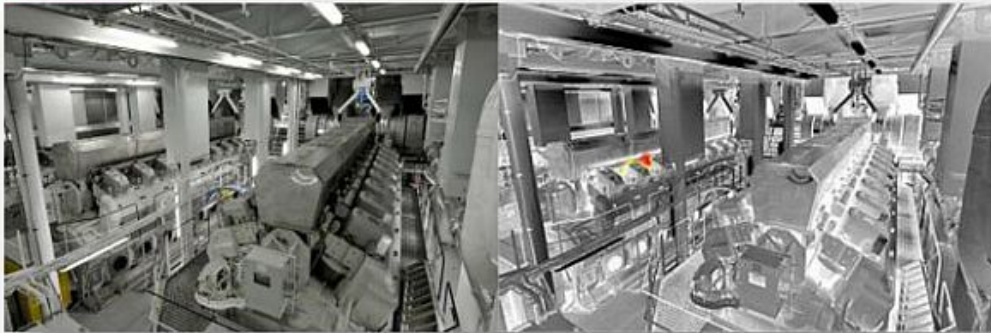
Flame Guard: Fire detection in a machine room
